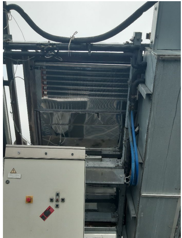
Figure 7: Backside of the collector with heat exchanger for the OPD.
