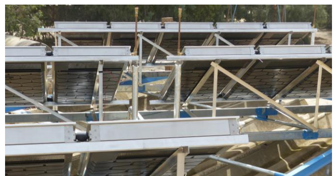
Picture 3: The back of the collectors showing collector-level overheating prevention
